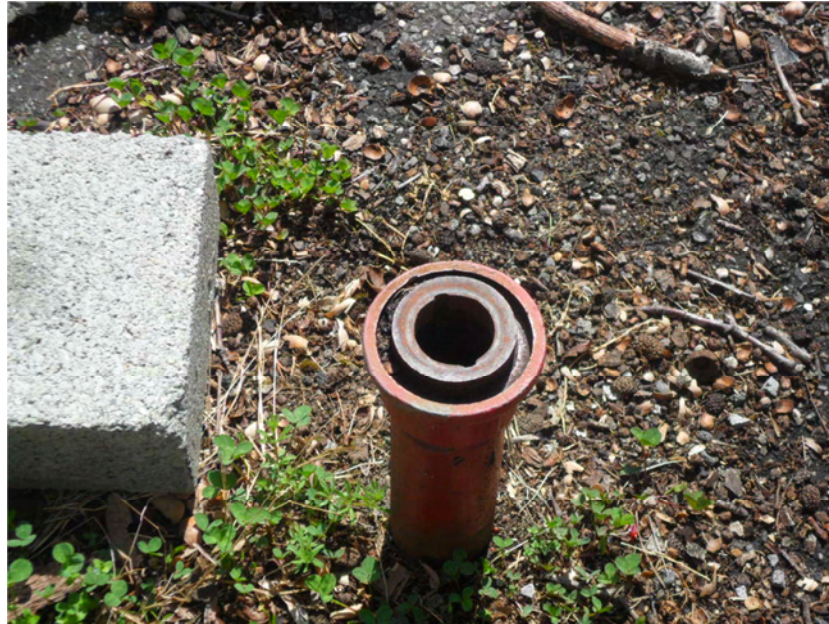
Photograph 53: Close-up of potential filler pipe
