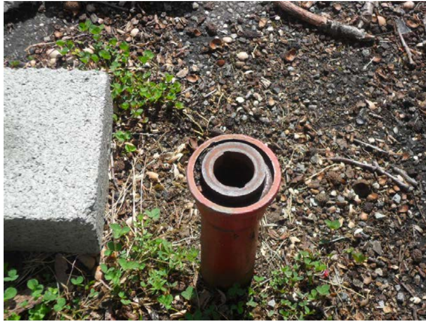
Photograph 29: Potential filler pipe located in the southwest corner of community center
