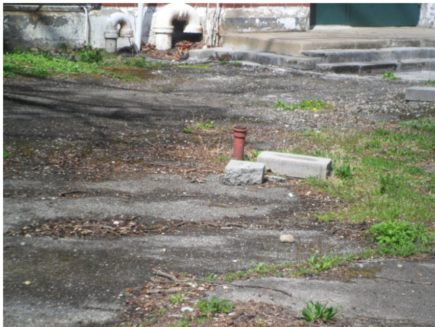
Photograph 30: Close-up of potential filler pipe
