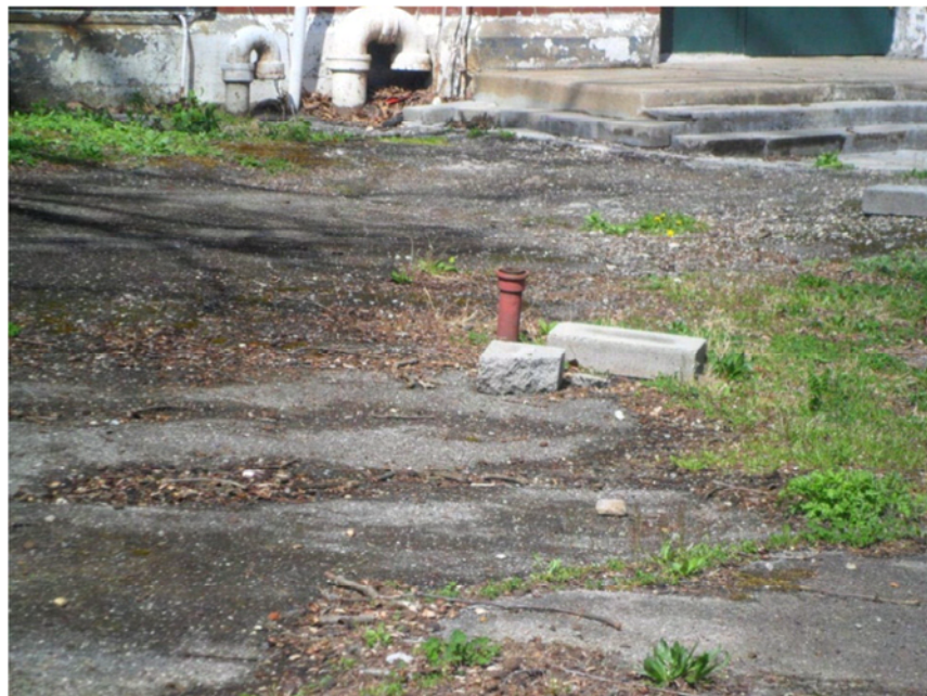
Photograph 52: Potential filler pipe located in the southwest corner of community center
