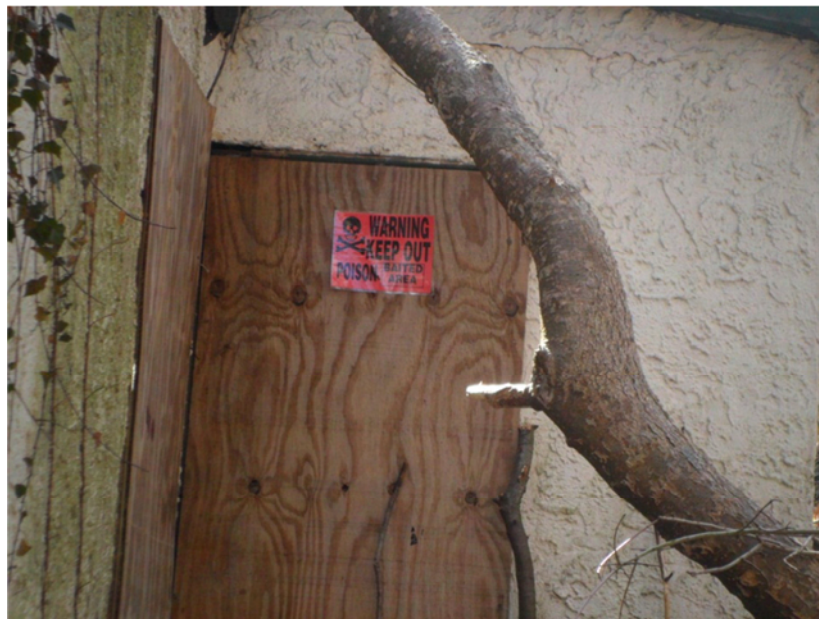
Photograph 24: Warning notice located on western perimeter of abandoned building
