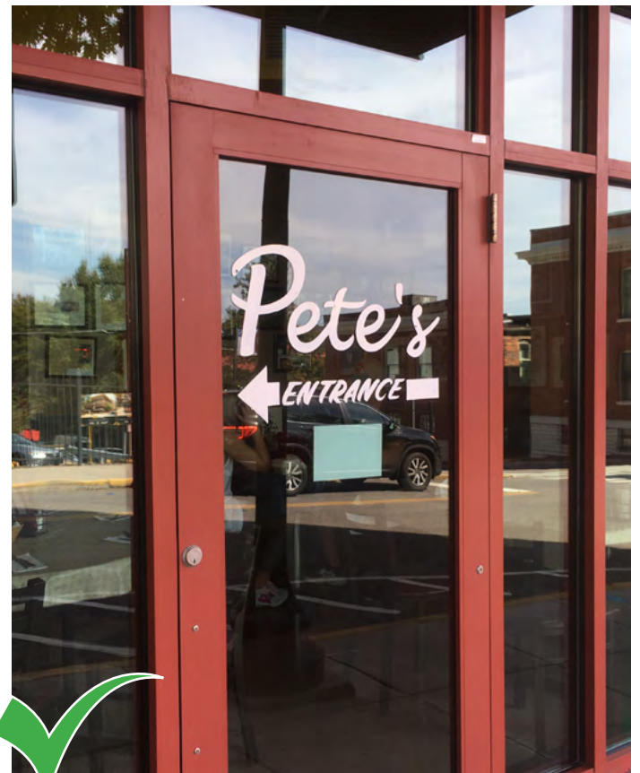
Do provide clear signage when doors are not in use.
